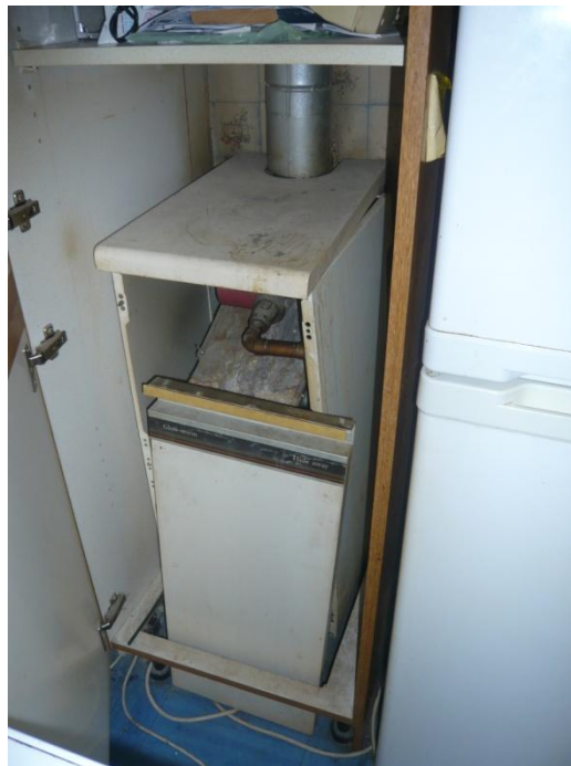
Figure 6 - Boiler in household 3 (Sally)
